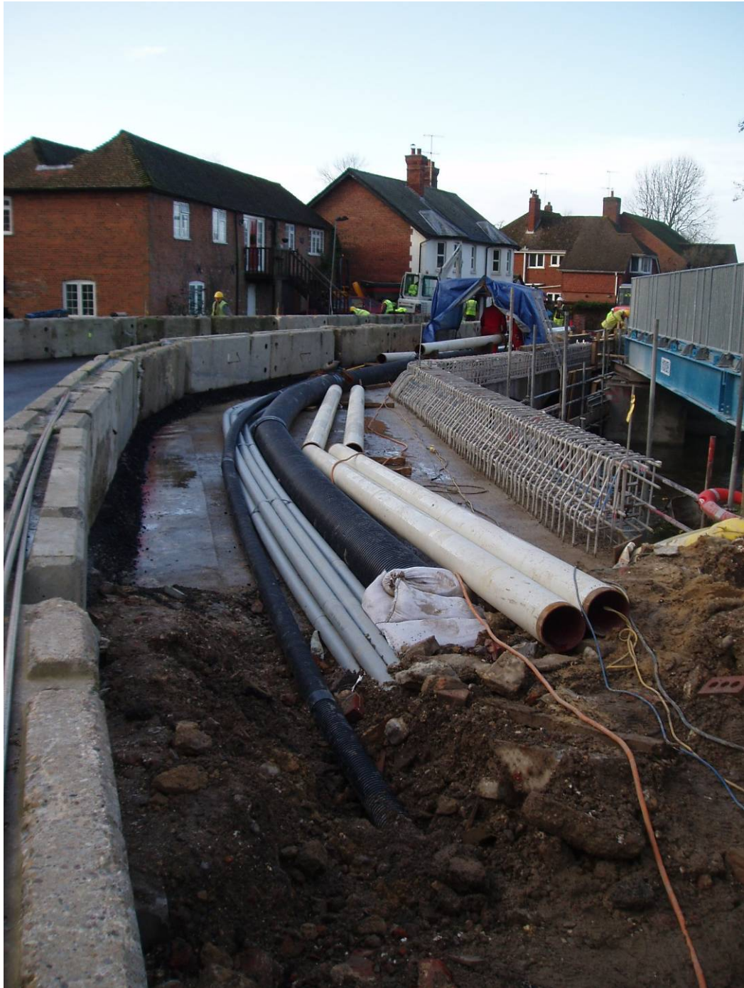
Photograph 3 Utility duct maze
