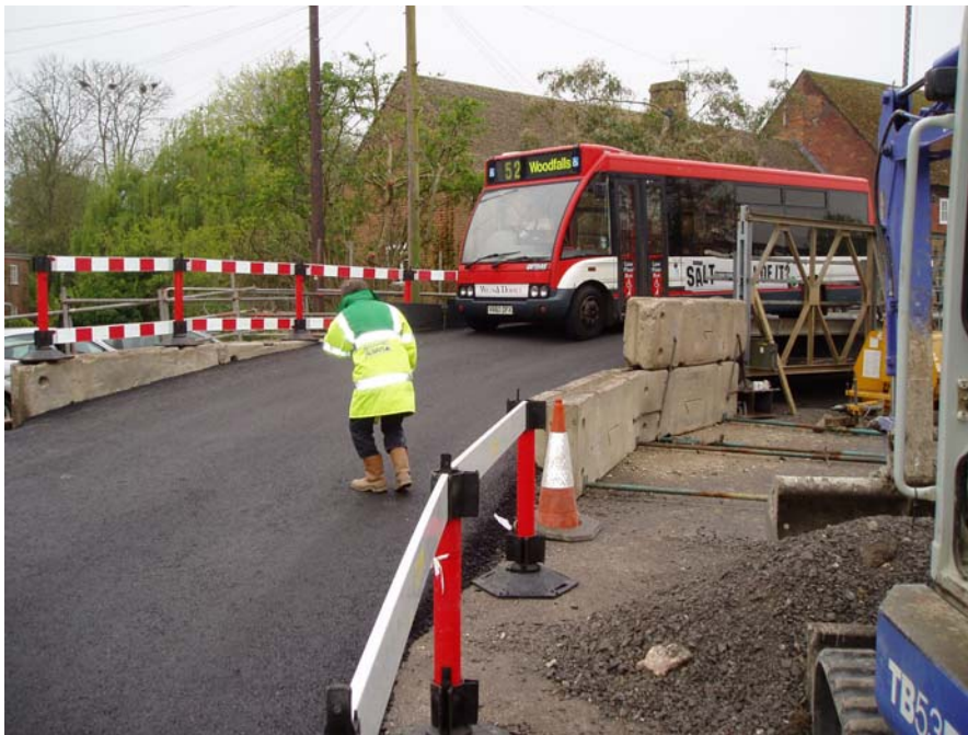
Photo 2 – Temporary vehicle bridge approach ramp (High Street end) ground clearance of buses.
